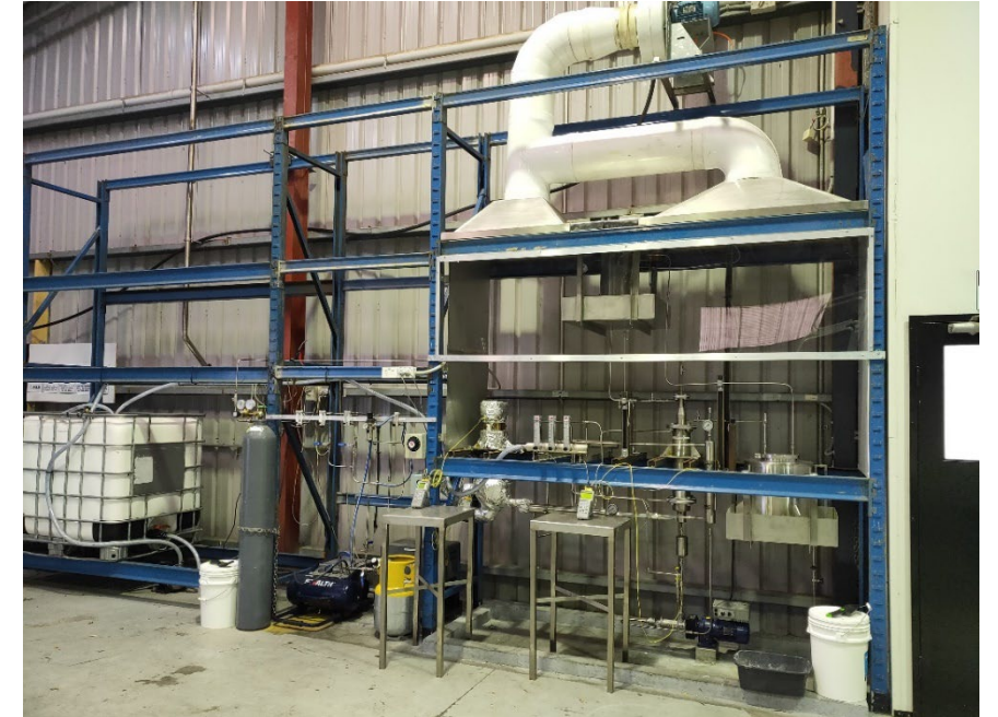
Oleum production plant
