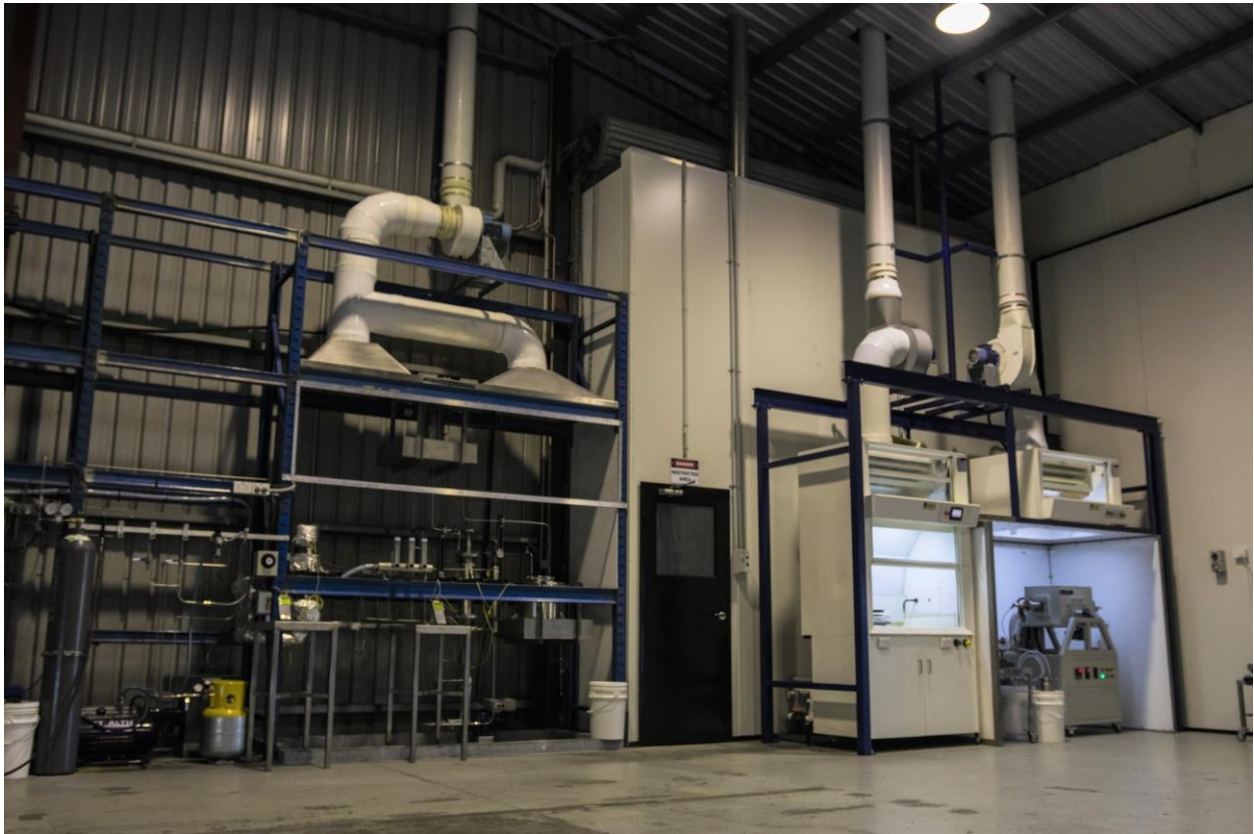
Figure 5: Section of the Alcore Technology Centre upgraded to allow the operation of three new laboratory reactors
