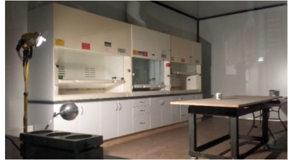
3 large fume cabinets for Lab test runs taking 7 to 20 minutes
