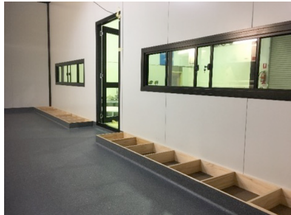
Flooring applied to kick-board bases of rear Core Lab benches and the door threshold sills for all 3 laboratory doors. Note that the windows are for external observers to monitor the lab work.
