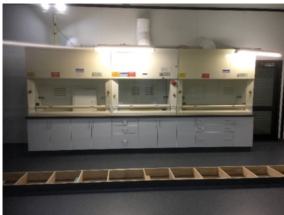
3 large fume cabinets are sealed and ready for wiring-up. Exhaust conduits will send fumes into a scrubber unit filled with water & neutralising lime water, thence into a collection tank for testing prior to release into the waste disposal system for the Berkeley Vale industrial park.
